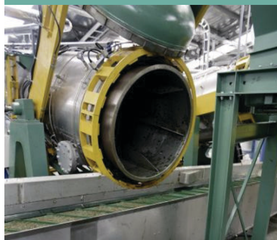
Figure 2. One of the Mediclaves at Interwaste's Seaview plant
